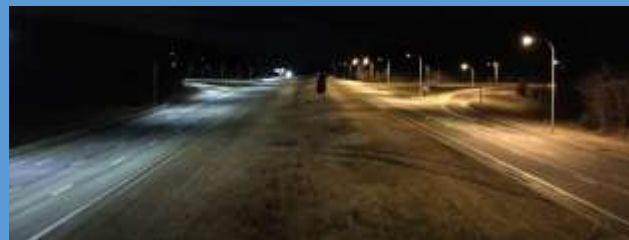
Streetlights on I-295 replaced with LED technology (on the left). Rhode Island is poised to become the first state in the nation to convert all State-owned streetlights to LEDs with control technology, with projected annual savings over $1 million. (Photo Credit: RIDOT)
